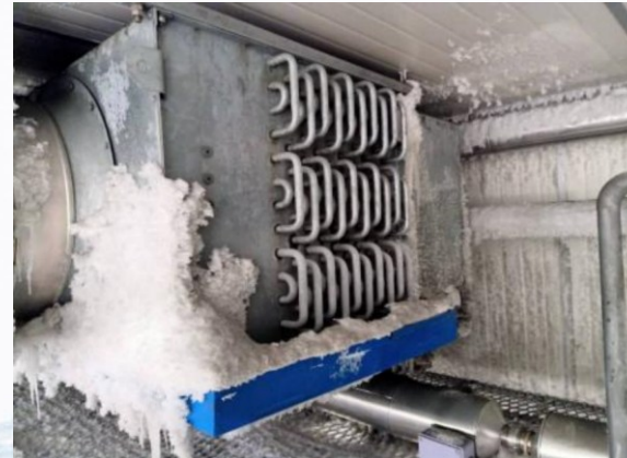
Pic. 2 – Excessive Icing on Evaporator
